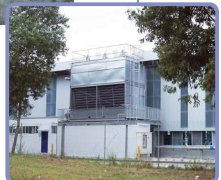
● Cooling equipment for noise reduction
