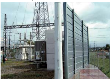
A soundproofing wall for a charging transformer
