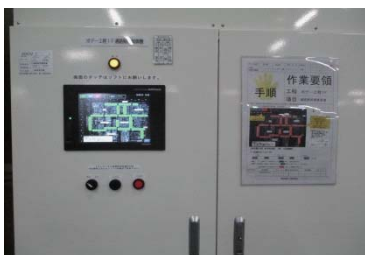
Central control panel for Inabe body process corridor lighting
